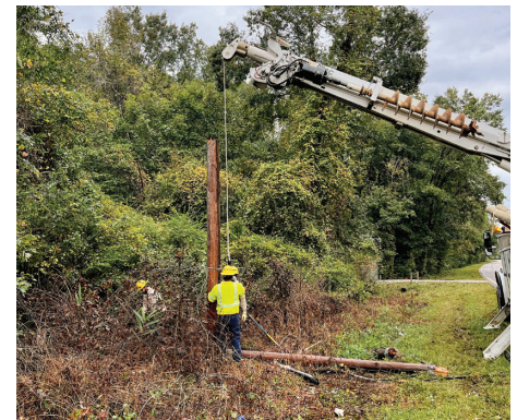
As soon as a storm subsides, Santee Electric crews are out making repairs to get power restored as quickly as possible.
